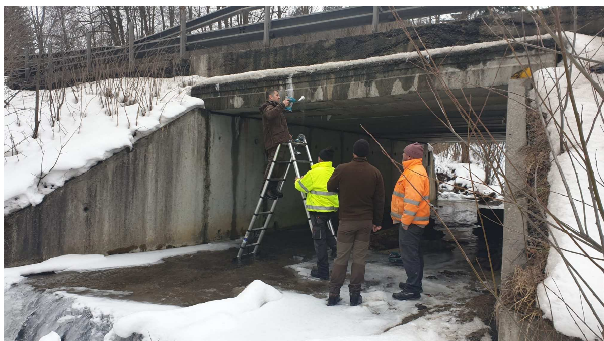
Figure 14: Installation of Reolink camera to monitor the adapted crossing structures in Romania.
