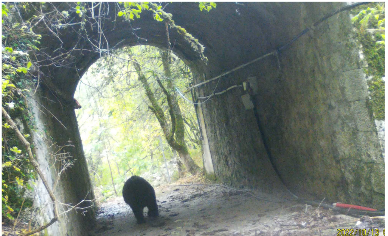
Figure 9. Bear detected at the improved culvert “Casone Antonucci” on the SS 83 road, PNALM.
