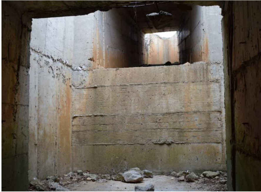
Figure 42. The culvert K73 had two vertical surfaces impermeable for the wildlife (photo L. Georgiadis).
